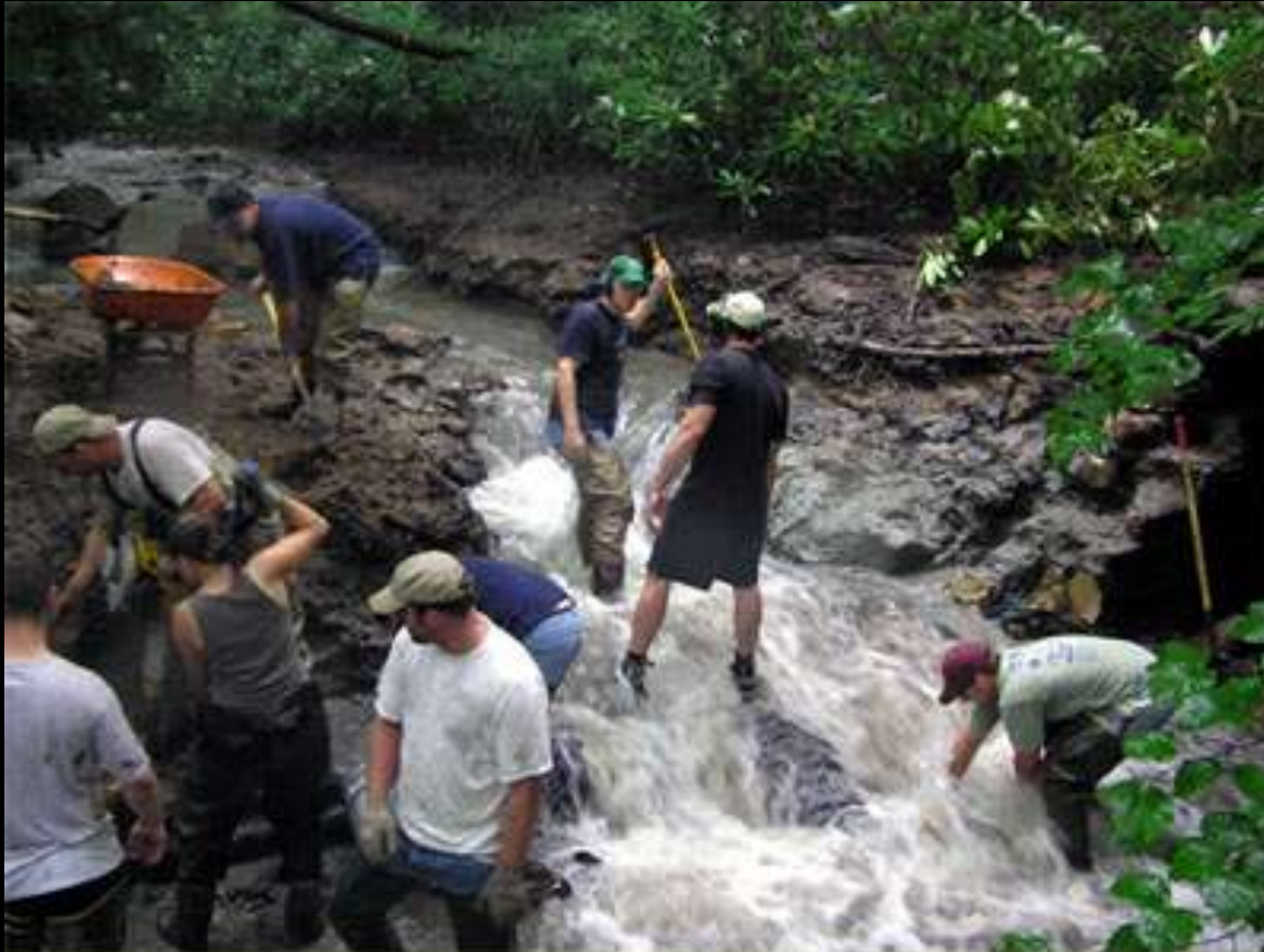
WPC staff members and partners brave mud and swift currents to remove a 25-foot-wide dam by hand.
