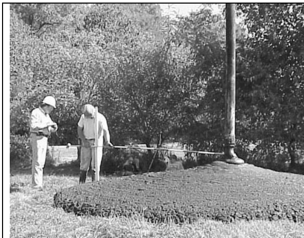
Figure 5. Sediment from both the concrete pump truck shown here and conveyor truck formed piles about two feet high. The equipment can be used to precisely place
