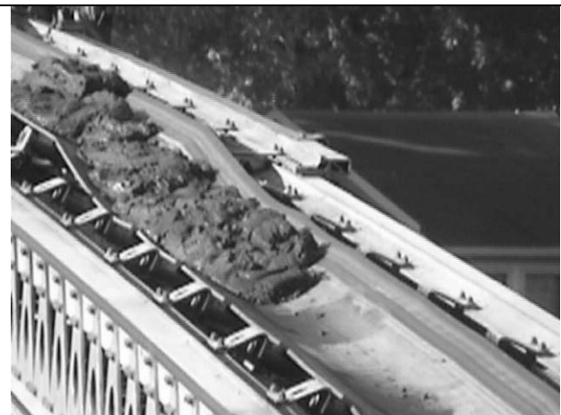
Figure 6. Excavated sediment had no difficulty on the conveyor belts. It rode inclines, passed through transfer points, and was readily cleaned by belt scrapers.
