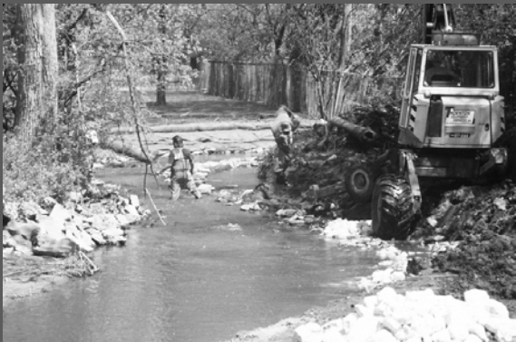
319 Project 97-08 Langendorf Pond Retrofit to Reduce NPS Pollution in the Flint Creek Watershed BMP-Stream Channel Restoration
