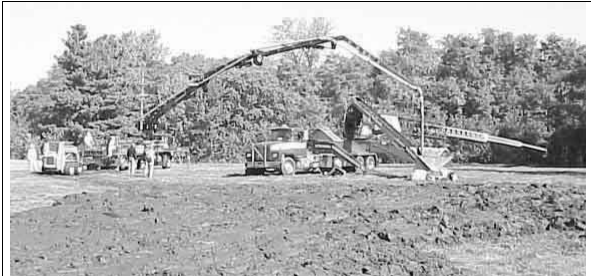
Figure 4. The site layout for the sediment handling demonstration at Lacon in September 2002, included a sediment stockpile in the foreground that was loaded to the pump truck on the left with a skidder. The material was pumped through a 32-meter boom shown here feeding the truck hopper. A feeder conveyor then carried material to the top of the conveyor truck where it passed through a transfer point onto the 105-foot telescoping main belt that placed the sediment on the field.
