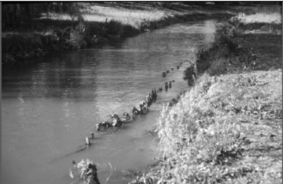
319 Project 93-05 Skokie River Restoration Project BMP-Streambank/Shoreline Protection. A fiber roll stabilization technique is used in this picture to protect the streambank.
